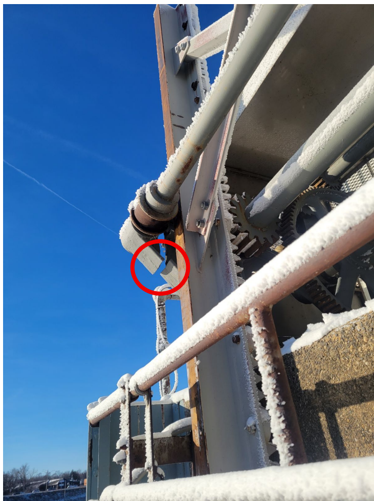
Figure 1 January 2024 Damage to South Sluice Gate Machinery; Temporary Repair has been Completed
