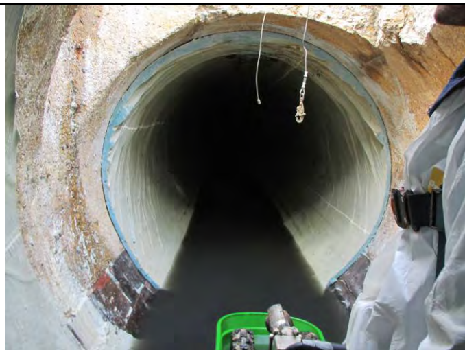
Liner terminating at a manhole. (Courtesy BGM)
