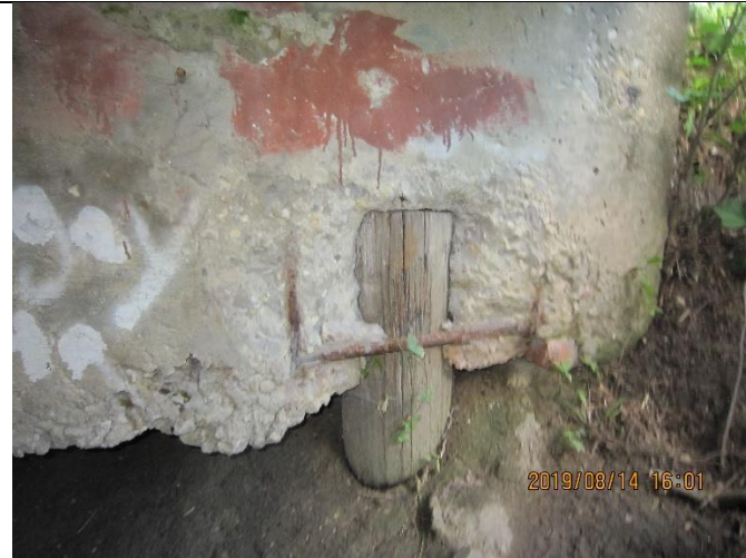
Photo 7: Concrete spall exposing timber pile and reinforcement.
