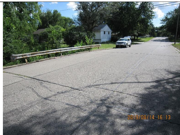
Photo 9: Longitudinal cracking through the wearing surface. Alligator cracking near the approach joints.
