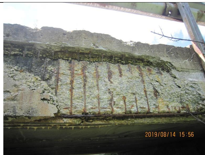
Photo 6: 5' x 1.5' Spall along the side of beam 11 with strands and stirrups exposed.
