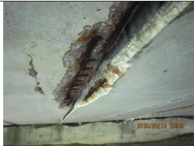
Photo 5: Edge spalling along Beams 9 and 10. Multiple strands and stirrups exposed.
