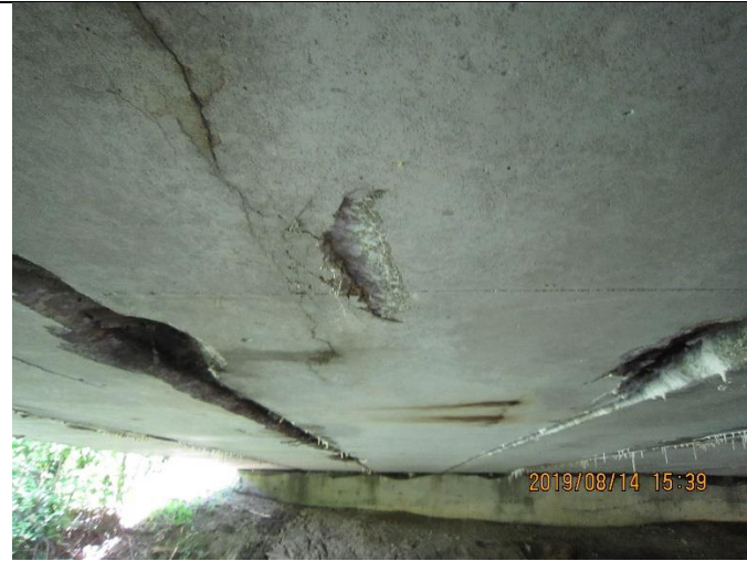
Photo 4: Longitudinal crack with delaminated concrete along Beam 9. Rust stains around the crack.
