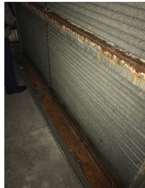
Chilled Water Cooling Coil and Condensate Drain Pan
