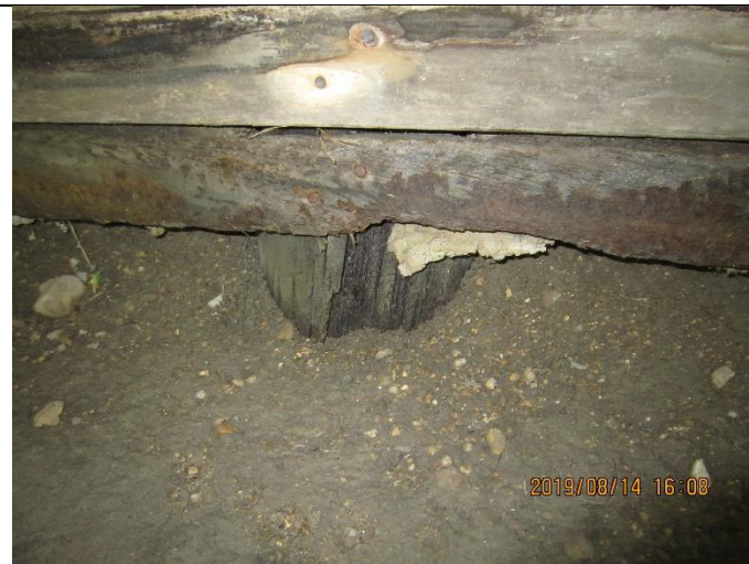
Photo 8: View of one of the exposed timber piles showing some decay.
