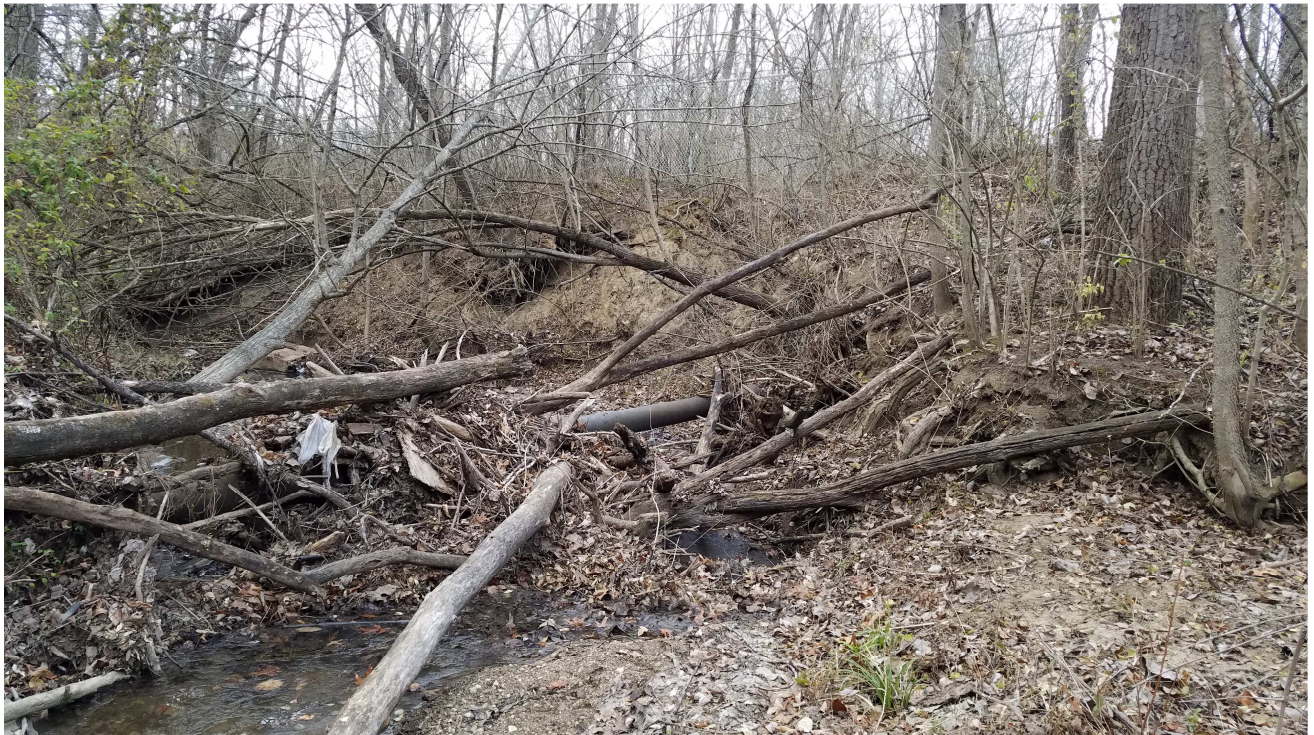
Photo 2: Faces downstream showing erosion and log jam around exposed pipe
