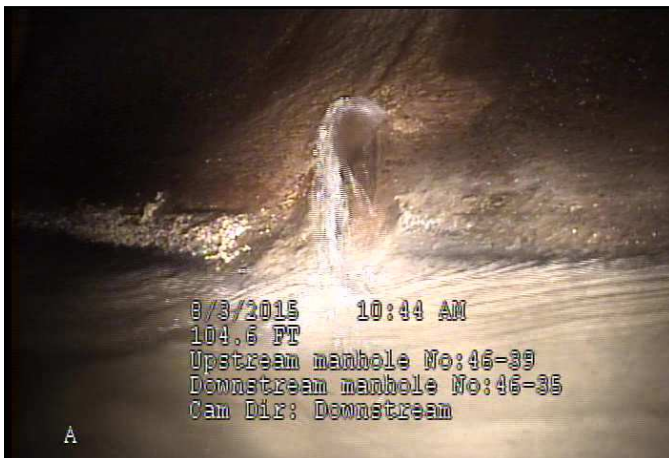
3. Infiltration at a deteriorated joint. Fairview Park.
