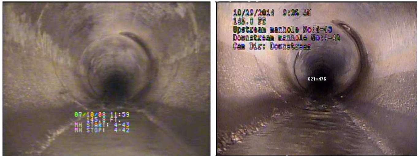
Figure 3. The view of the McKinley Sewer on Kellar near Central taken in 2008, (on the left) is brought into much better focus using high definition inspection cameras now available (2014 image on the right). Flow line erosion and infiltration stains are readily visible.
