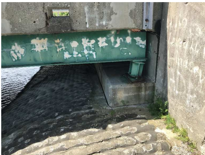
Rockers on West side appear to be over rotated.
