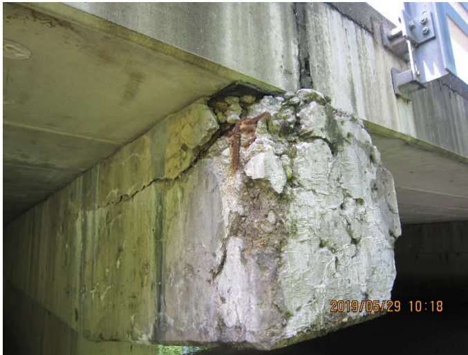
Delamination and spalling on north end of east pier.
