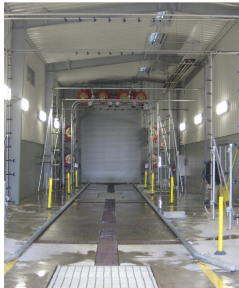
FIGURE: 7 DRIVE THROUGH TOUCHLESS WASHER
